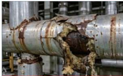
손상상태 (Damaged Condition)
